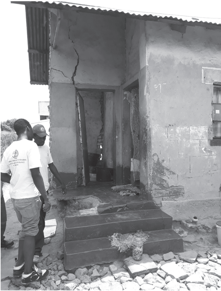
Figure 9.4 Cracked houses in Mufulira. Photograph by the author.
