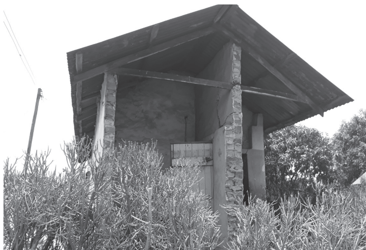
Figures 9.3 Cracked houses in Mufulira. Photographs by the author.
